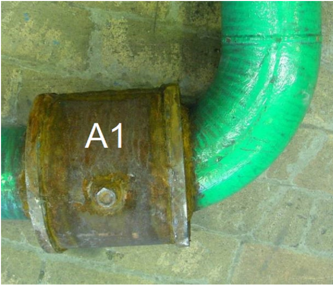
Fig. 3. A1 joint of the high-pressure ammonia water pipeline
