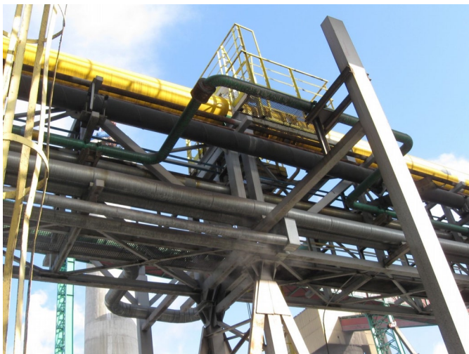
Fig. 1. View of a part of the ammonia water pipeline
